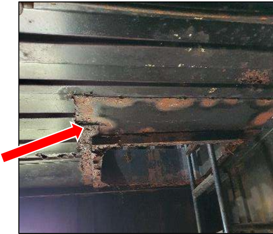
Lantai Smoke House Aras 1 Berkarat PULAMAR, Johor (29.09.2020)
